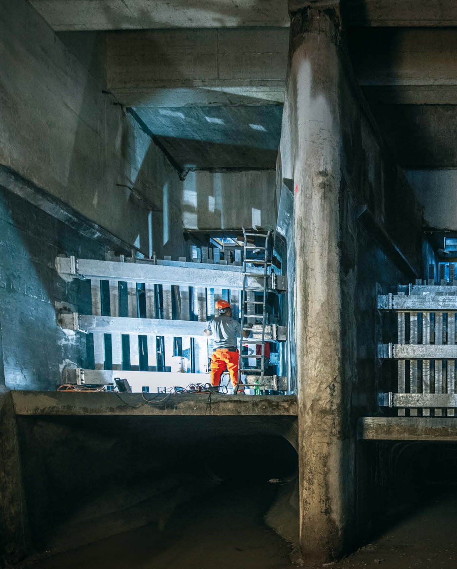
The rails in the energy dissipation structure downstream of the synchronous discharges have been completely replaced. These elements help to dampen the pressure of the water exiting the synchronous discharge before releasing it into the discharge channel.
